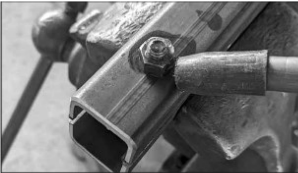
Fully weld the nut in place. It may take a minute before you can un-thread the bolt
