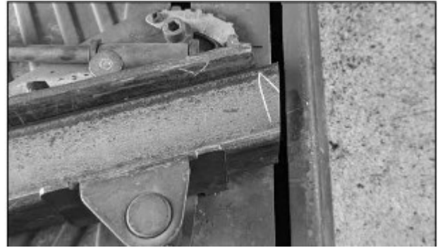
Cut the end of all the legs to 15°. The cuts are parallel not opposite. Weld seam up or down
